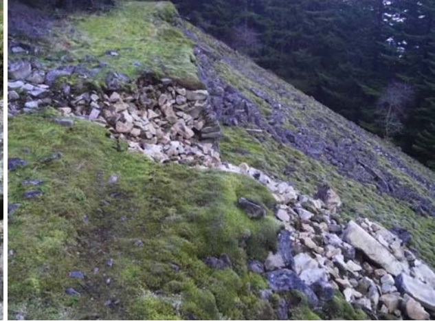
Figure 43. View west of recent wall collapse.
