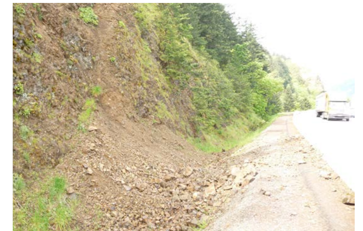
Rockfall along I-84.
