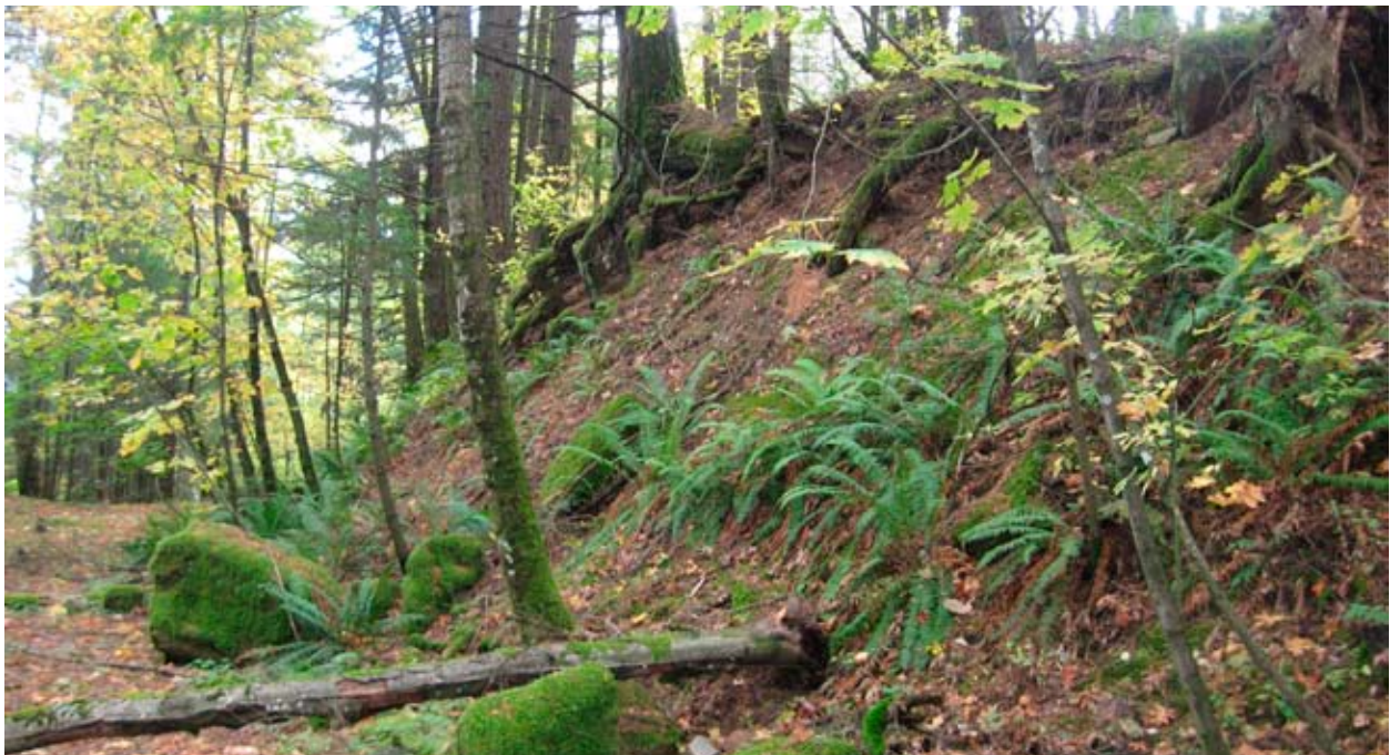
Cut-through, Lindsey Creek Segment. The eyebrow of this cut is compromising the trees and integrity of the slope. Fallen rocks and vegetation are also damaging.
