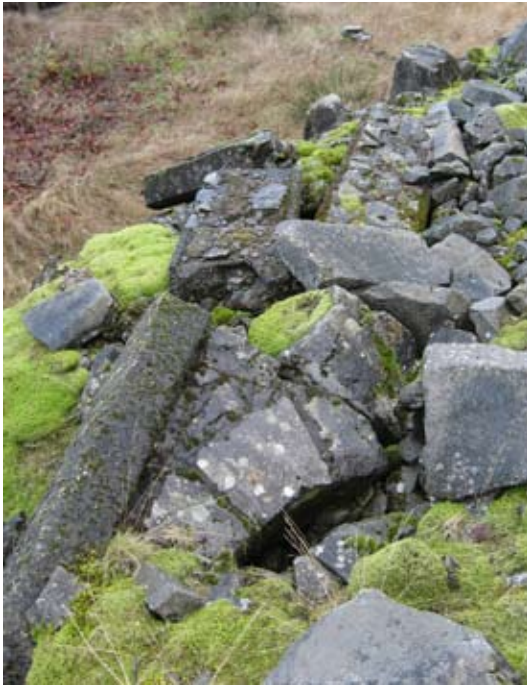
Broken parapet, Shellrock Mountain
