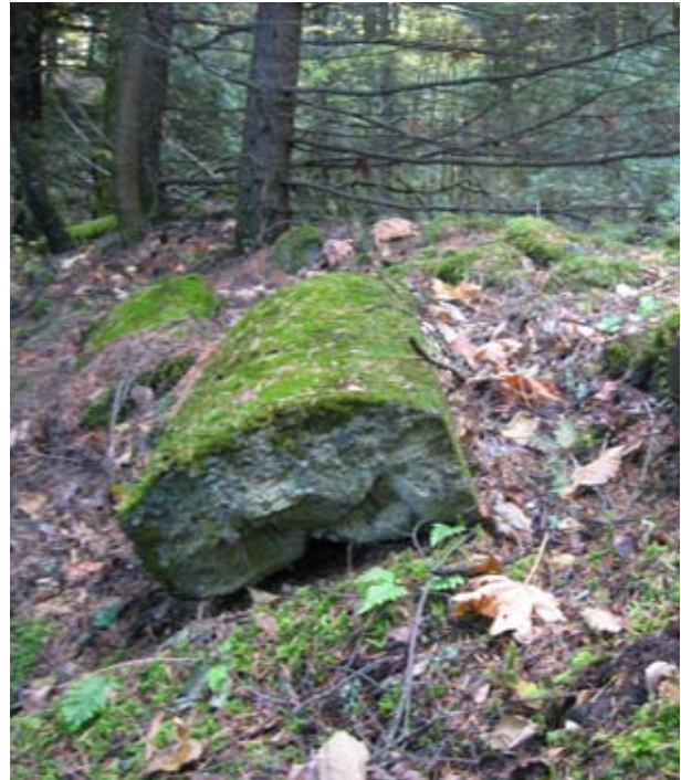
Collapsed Masonry Parapet, Lindsey Creek
