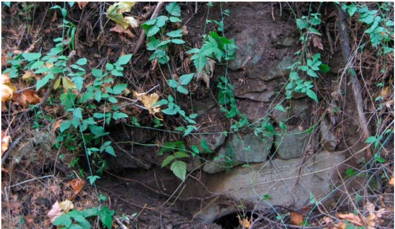
Clogged concrete culvert, Mitchell Point Segment 2
