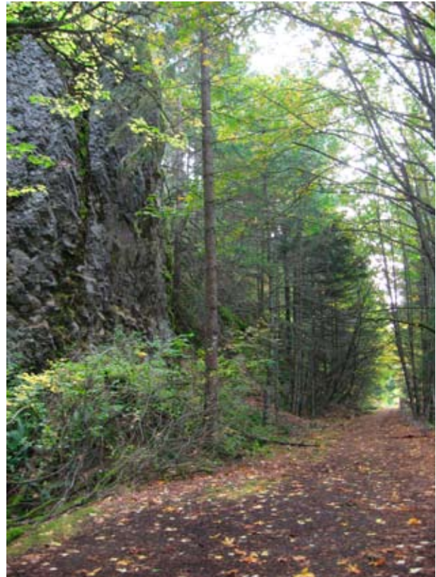
Cabin Creek area, Starvation Creek Segment. Overgrown vegetation along road edge, slide (right, background), debris and mud build up on edges of the road surface.
