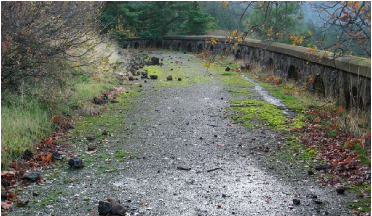
Reconstructed and repaired rubble masonry parapet, damaged and partially buried roadbed, Ruthton Point
