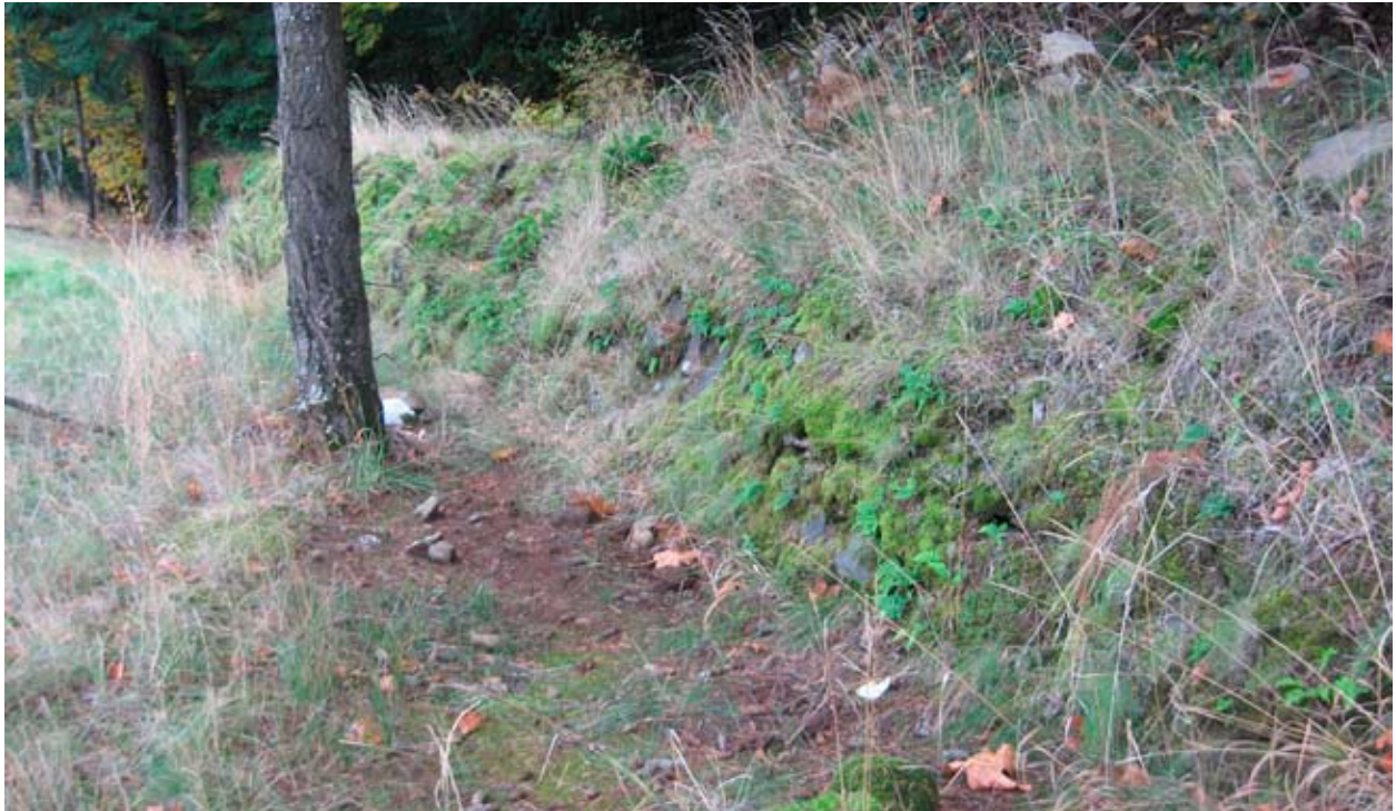
Retaining wall north of Historic highway. This may be part of a longer wall. It is damaged by the ferns and other vegetation, missing chink stones.
