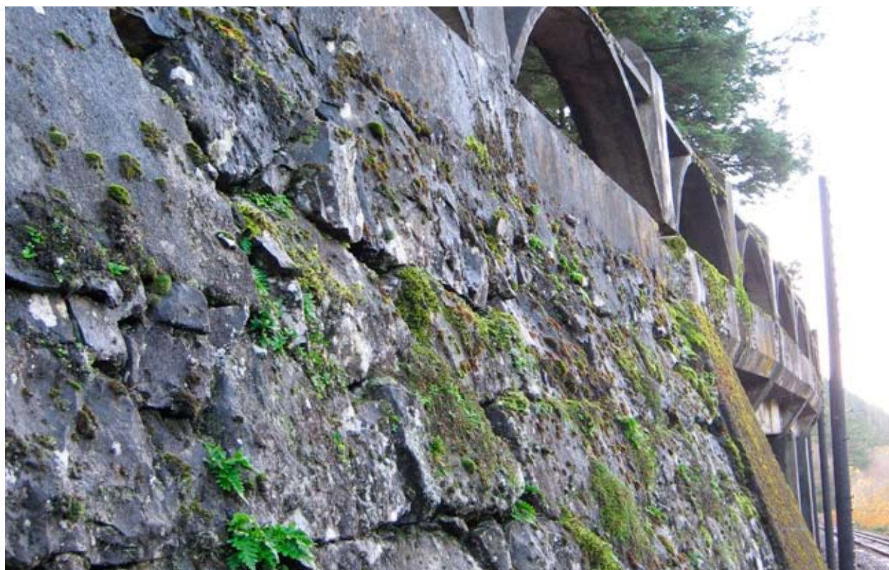
Retaining wall, viaduct and guard rail, near Multnomah Falls. The retaining wall is battered (sloped to the base), dry laid, unbossed, and laid in a random pattern. Many chink stones are missing, some can be seen.
