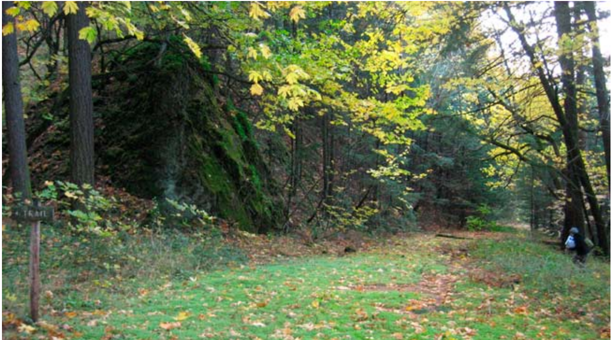
Mitchell Point Segment 2, Wyzant trail intersection. Overgrown pavement, clogged drainage system.
