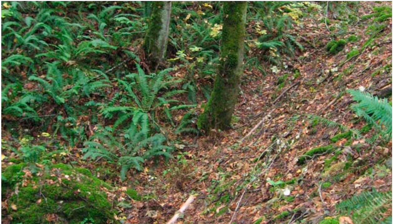
Fill-through, blocked drainage, Lindsey Creek Segment
