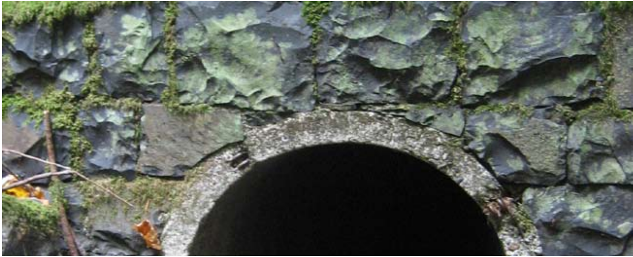
Cabin Creek culvert detail. The basalt stones on this culvert would be described as medium sized, hewn, bossed (shaped to have a convex face), laid in straight courses, dry laid with mortar around the pipe.
