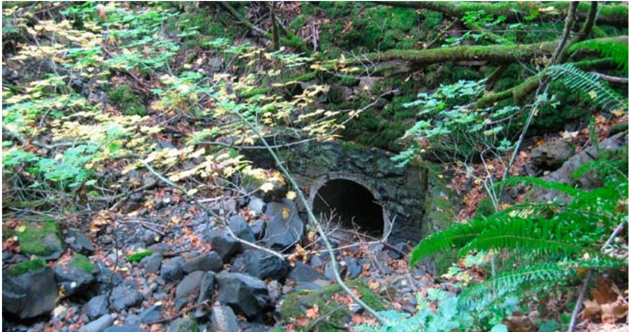
Cabin Creek culvert. The style of this culvert suggests it was meant to be seen from a path to the fall.
