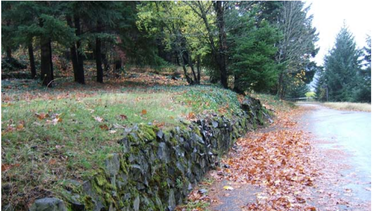
Mitchell Point Segment 3, retaining wall and settlement site from parking lot. The wall has failed and been patched with mortar and rubble.
