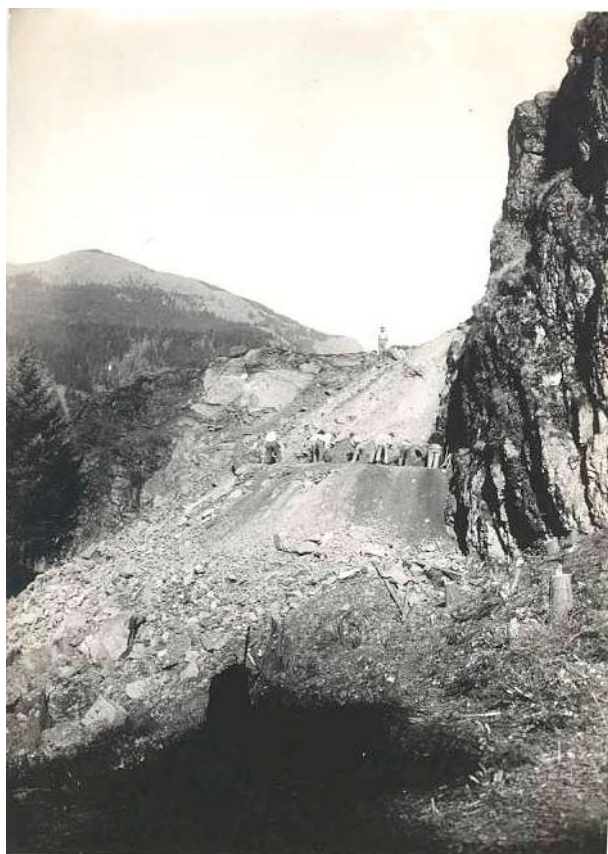
Constructing the Hood River County section, forty eight foot rock cut and forty foot fill. From Elliot 1914.
