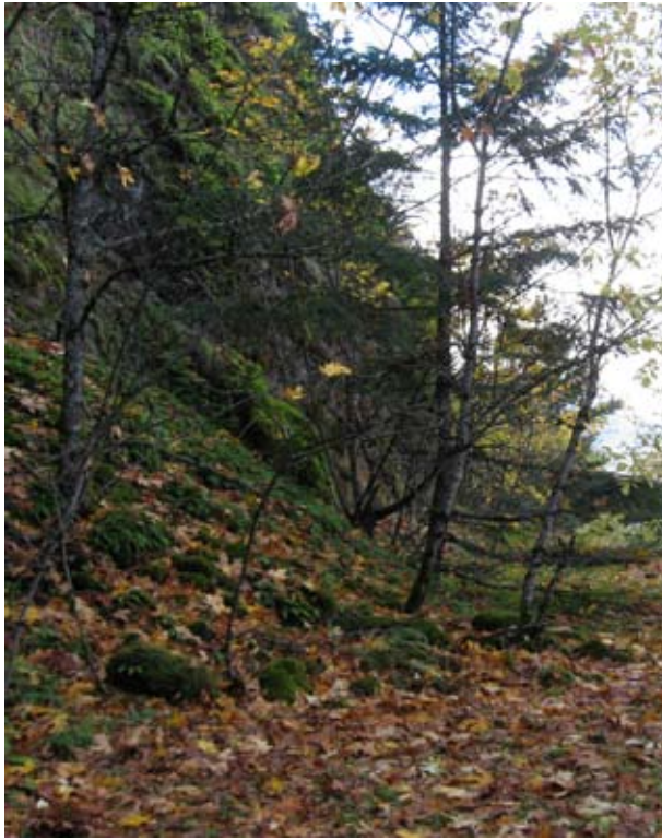
Rock cut, slide, Perham Creek
