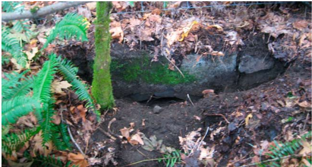
Buried, clogged culvert, Starvation Creek Segment
