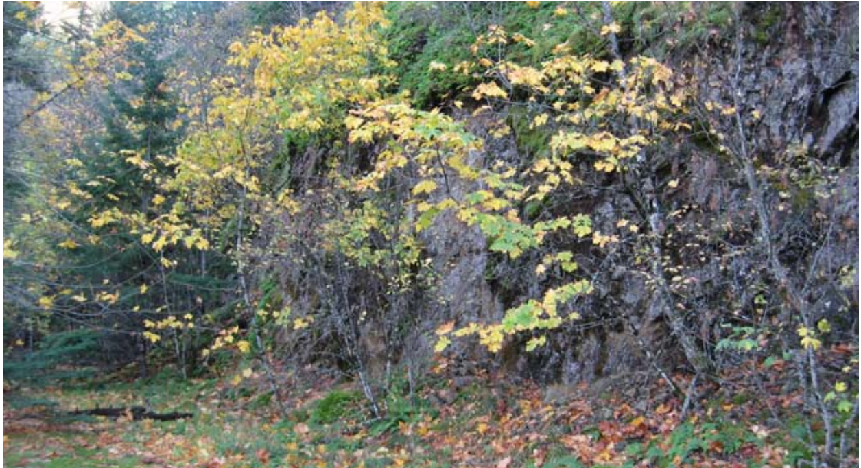
Rock Cut, Mitchell Point. The vegetation and piled debris at its base are signs of poor condition. Note the slide in the background.
