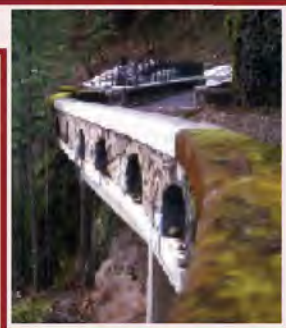
Picture right: The Eagle Creek Viaduct was damaged by a rockslide and as part of the project it was repaired to its original condition.
