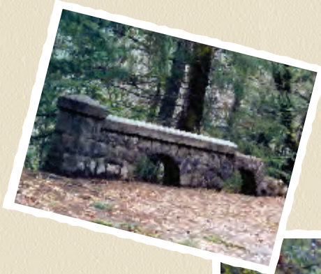
A view of the deterioration of the rubble masonry parapet walls on the Ruckle Creek Bridge.
