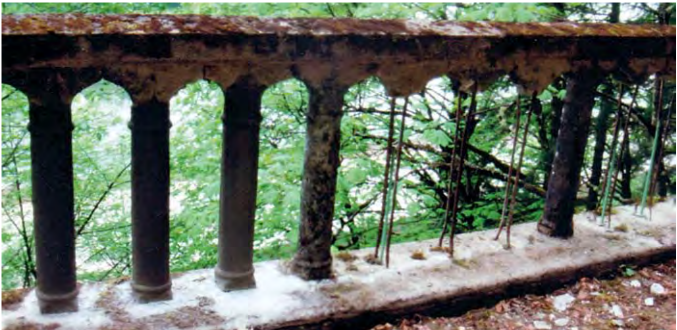
Figure 79—Toothrock Viaduct Railing deteriorated Condition
