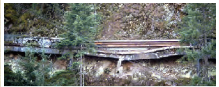
Many of the original viaducts and bridges have fallen into disrepair requiring, in some cases, major renovations and others replacement of the structure. The photograph at right is the old Eagle Creek Viaduct
