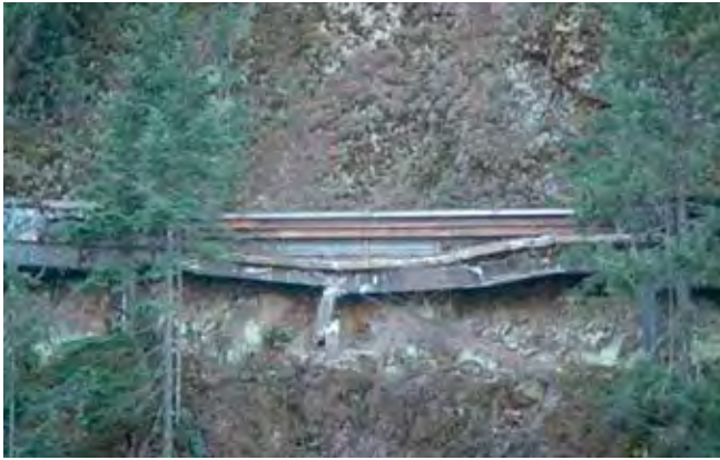
Figure 80—Damaged Eagle Creek Viaduct
