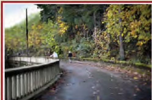
The deteriorated railing on the Toothrock Viaduct was restored to its original condition as part of the project.
