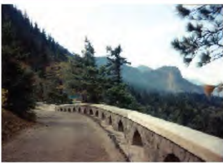
The viaduct railing and rubble masonry parapet wall have been restored in the section of the old highway alignment that skirts Ruthiton Point (highlighted in bold yellow dashed line in aerial at right.)
