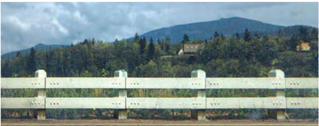
Figure 61—Two-Rail, Steel-Backed, Wooden Guardrail
