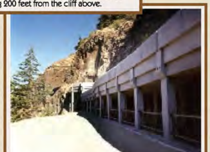
Fascia panels and the colored concrete were included as part of the design of the rock catchment structure to lessen visual impacts.
