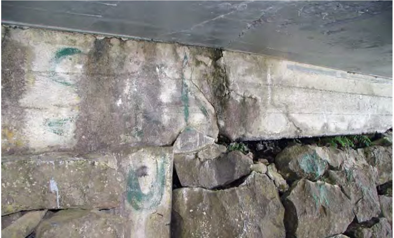
Figure 77—Deterioration of the Crown Point Viaduct
