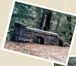
A view of the deterioration of the rubble masonry parapet walls on the Rucklee Creek Bridge.
